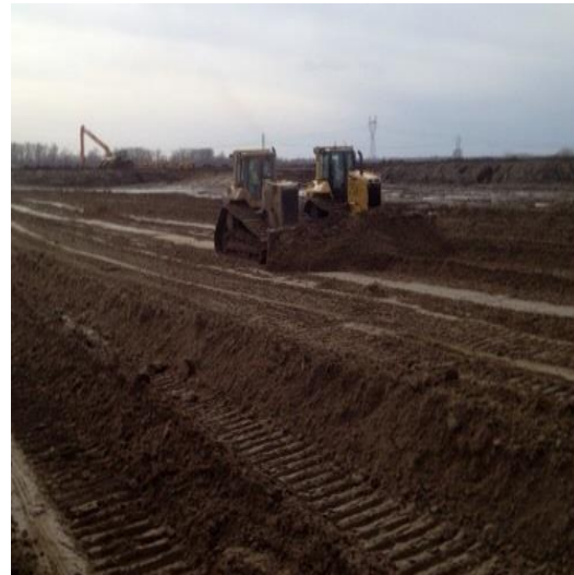
(C & M dozers working in unison to fill the breach area on Consolidated North)
